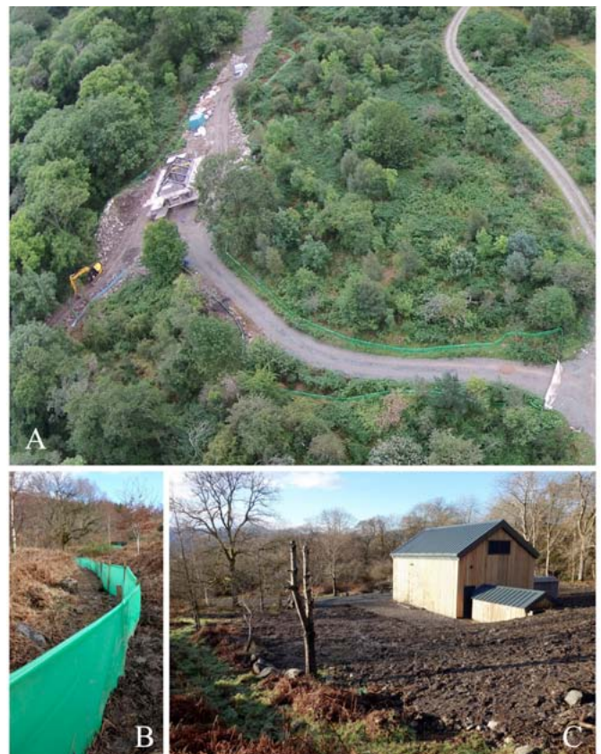
Figure 2. A Loch Lomond hydroelectric development. A. Aerial view of the lower section of the site, similar to that shown in Fig. 1, August 2014. The fenced area encompassing the construction site, with powerhouse containing the turbines, the cleared areas where the pipes had been laid, and the movable heavy sheet 'gate' placed across the access road, are apparent. B. Reptile-proof fencing that surrounded the construction area, February 2014; this was 50 cm high and included 10 cm beneath the ground. C. The completed powerhouse, with reptile fencing removed, November 2014.
