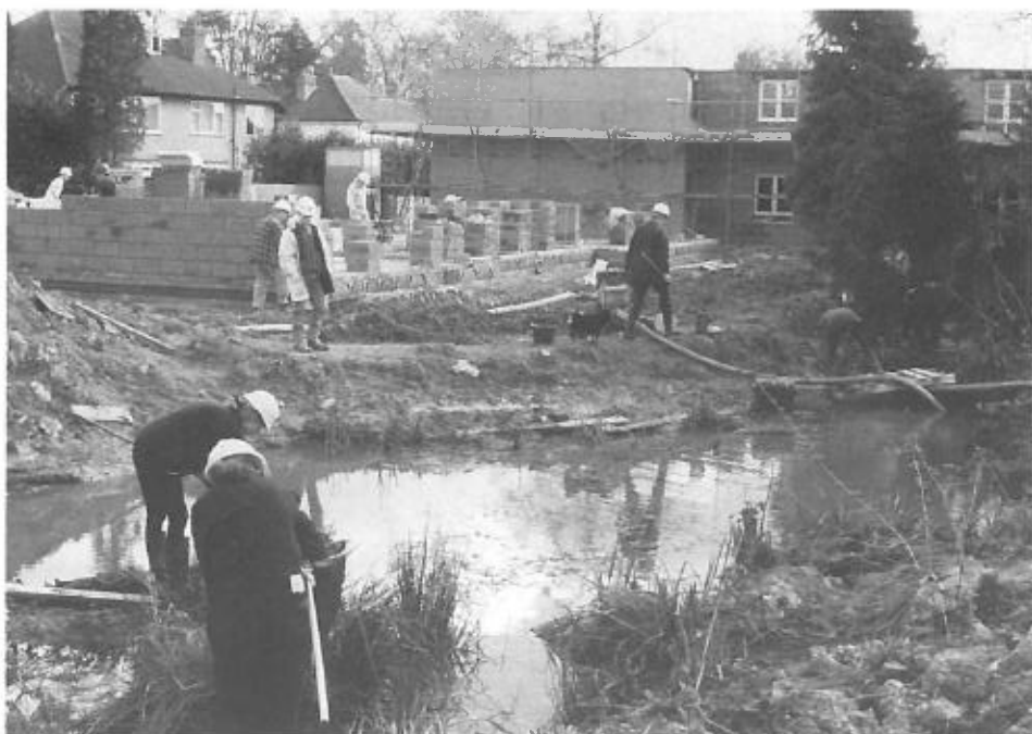
Plate 3. - Midway through the pond drainage, a few days later the same area was buried under concrete and brick, but hopefully all the newts had been safely translocated.
